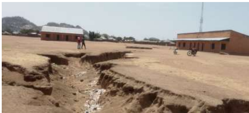
Plate III: Impact of gully erosion on school environment at Gombi 2
