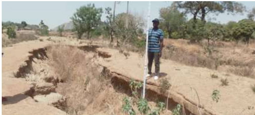
Plate IV: Impact of gully erosion on rural road along Fota
